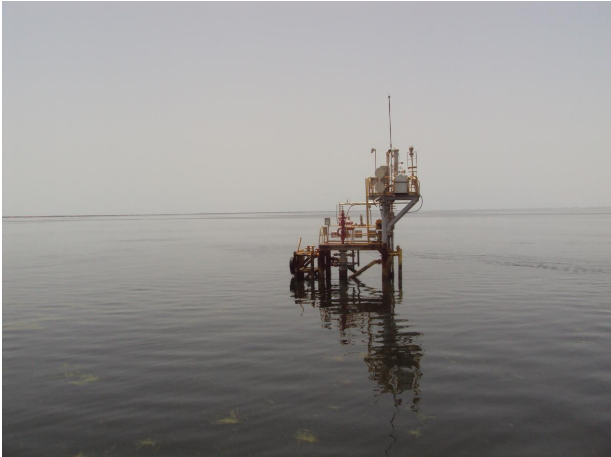
Figure All.1: Cercina 3 Wellhead
